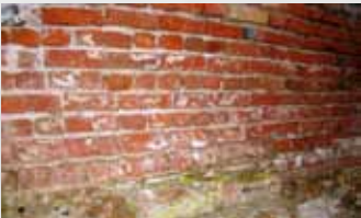
Kolodvar, 13. st. – zidina, način slaganja opeka u zidu (1 red vežnjak, 1 red dužnjak i 1 red vežnjak) Kolodvar, 13th century – method of bricklaying within the wall (1 course stretcher, 1 course header, 1 course stretcher)
